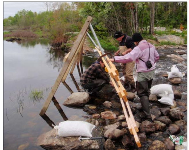
Robert Hogg (UMaine AFS), Tara Trinko, and Trent Liebich (both NOAA Fisheries) constructing an Alewife monitoring weir on Sedgeunkedunk Stream.
